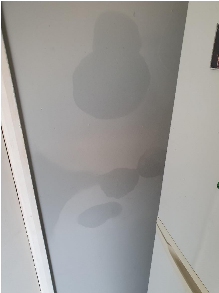
Signs of damp on internal wall between lounge and kitchen
