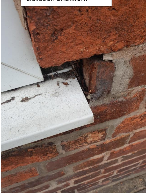
Repairs required to front elevation brickwork
