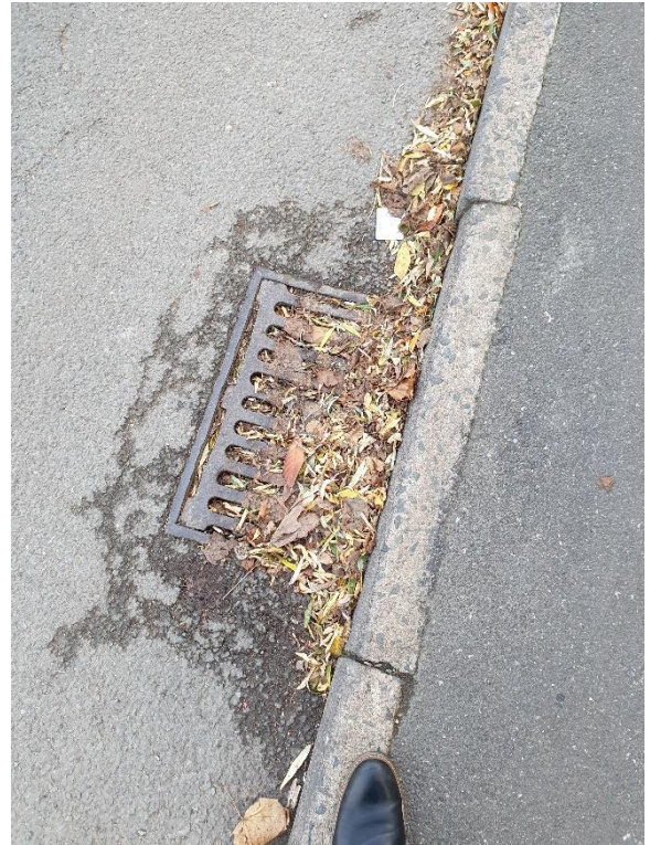
Blocked main drain on road
