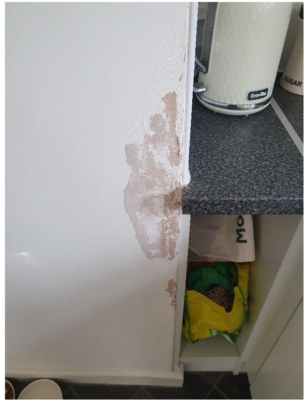
Damp to chimney breast in kitchen, previous works to chimney and DPC have been done
