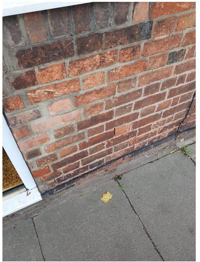
Repairs to front elevation, but more required
