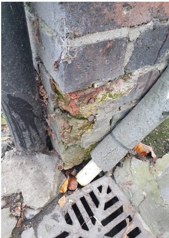
Front corner of property where water enters dining room
