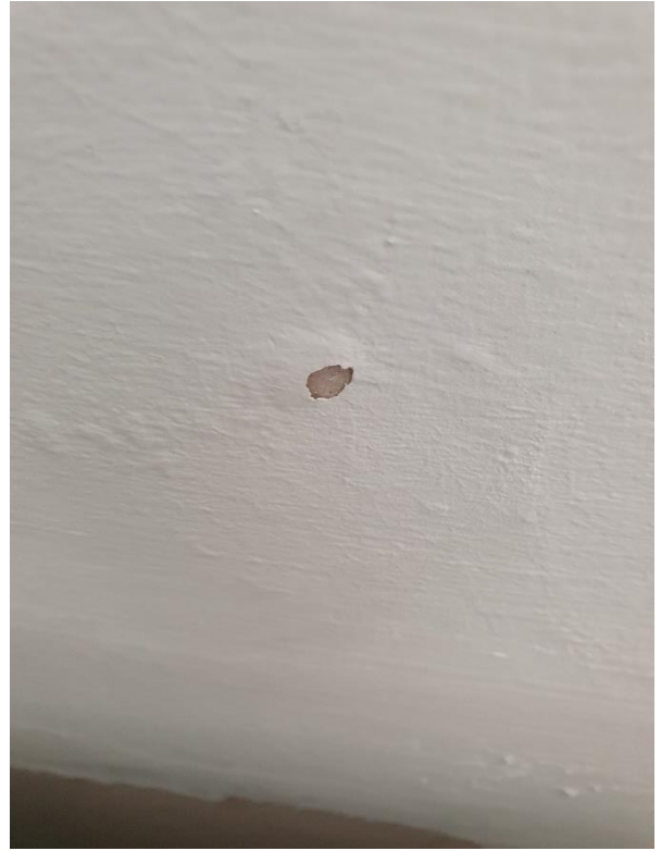
Peeling paintwork in kitchen
