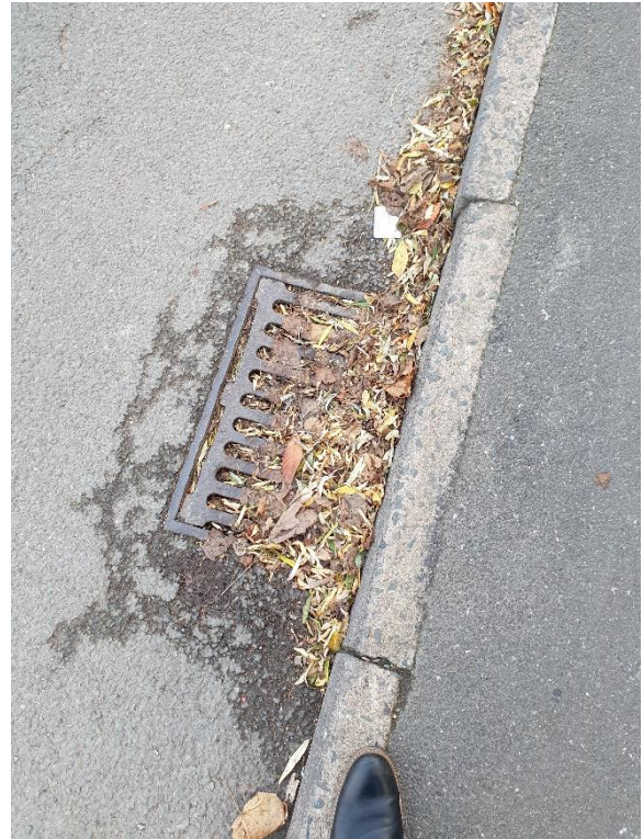
Blocked main drain on road
