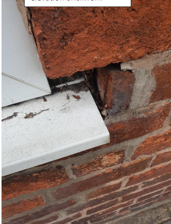
Repairs required to front elevation brickwork
