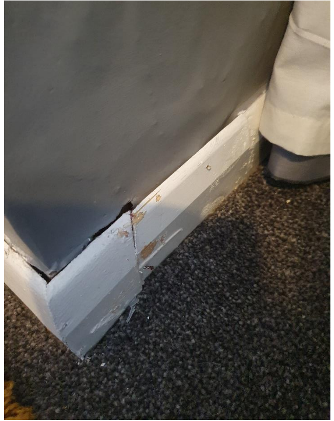
Damp to wall right of front door in lounge
