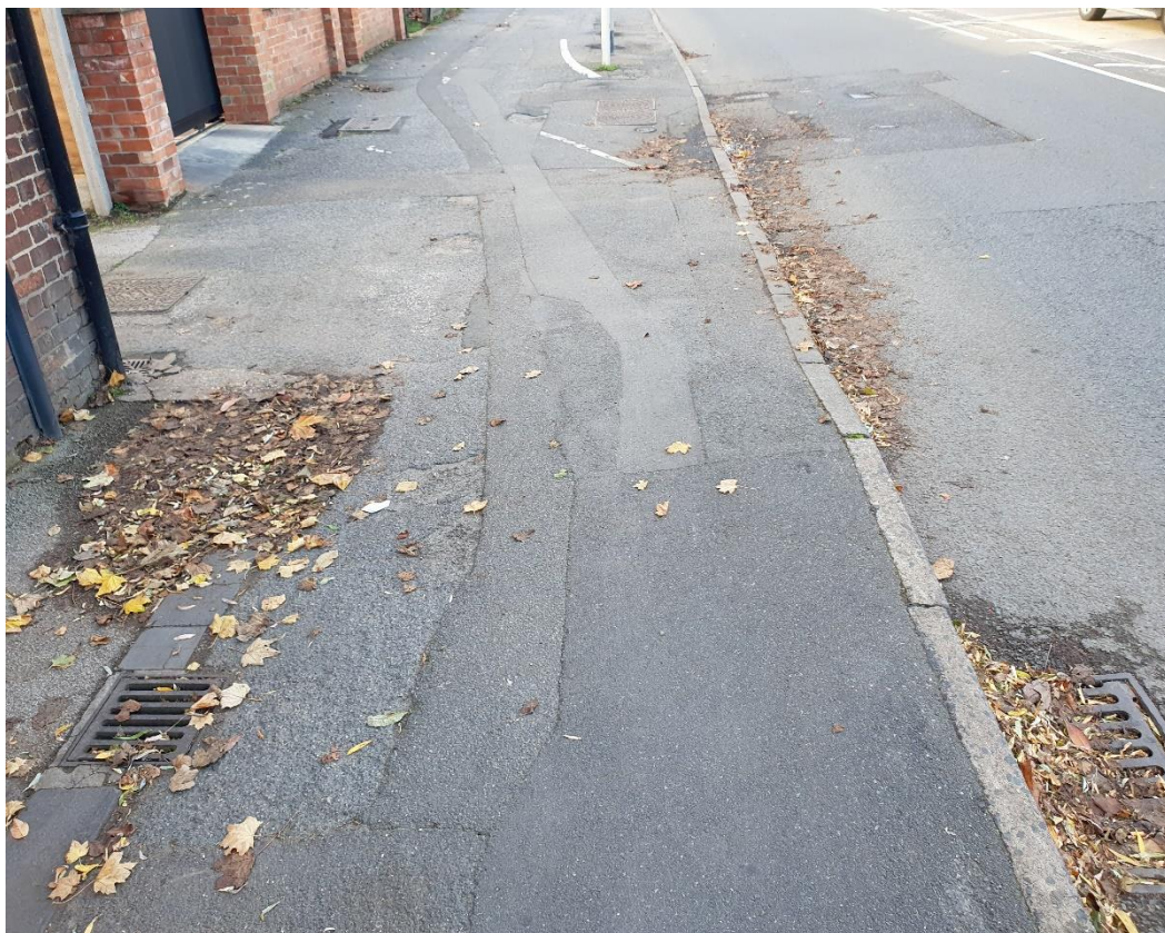
Photo of road runoff area
