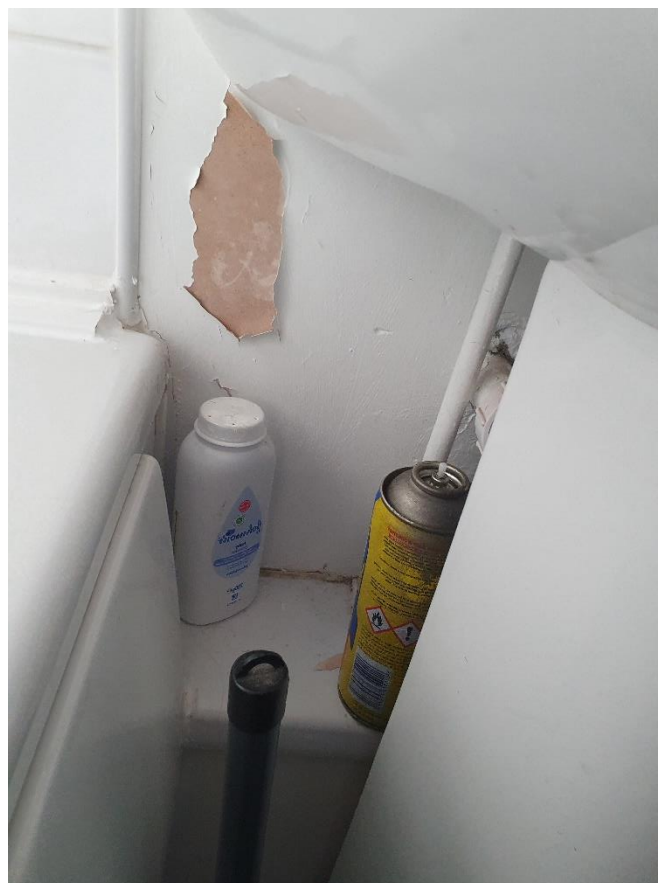
Damp area in bathroom possible condensation
