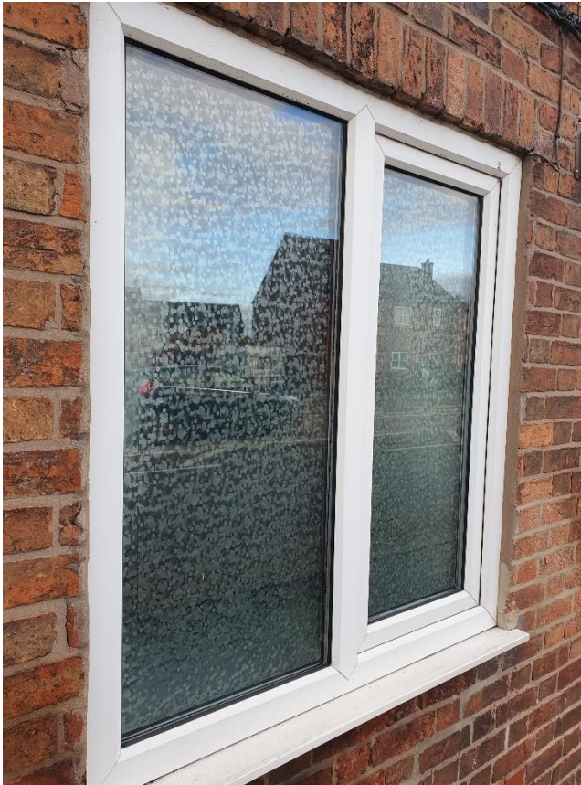
More evidence of sub-standard windows
