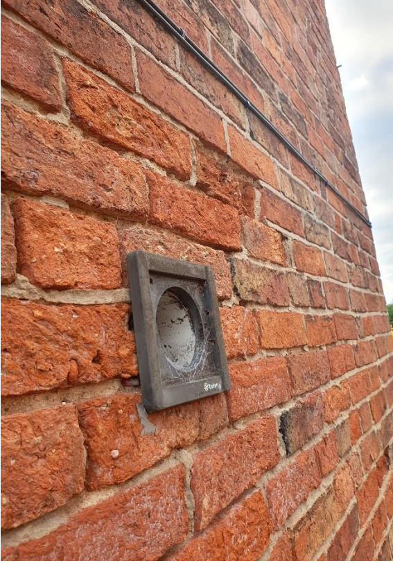
Missing vent cover and spalling brickwork to side elevation
