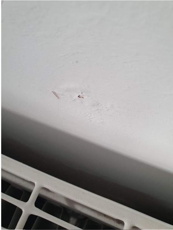
Peeling paintwork in kitchen
