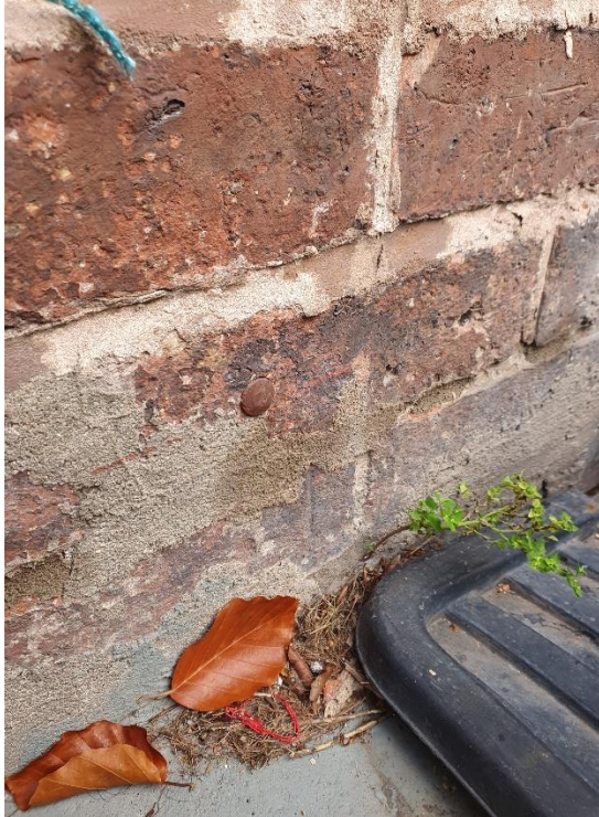
Evidence of historic DPC
