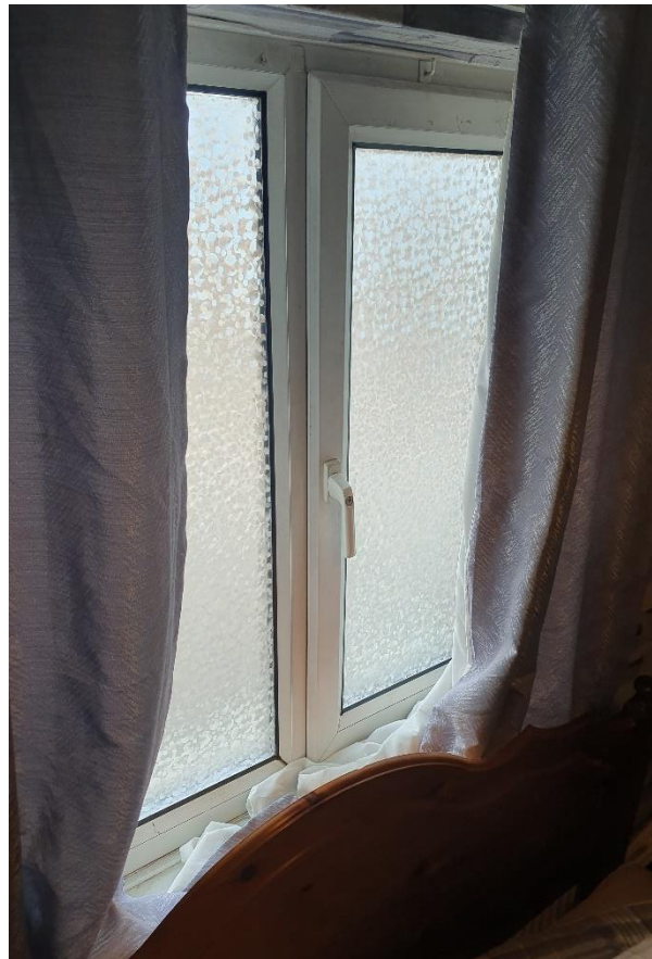
Opening inwards windows with no trickle vents
